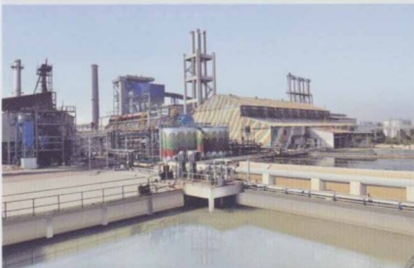
Sanghi desalination plant.
